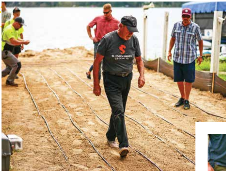
◀ Dan Wickham, center, inventor of SludgeHammer, walks the drip field during the educational outing for the Paw Paw job.
